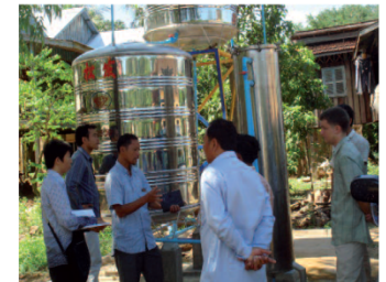
Implementation of a system in Po Ta Pang site in Kandal province in Cambodia, October 2011.
