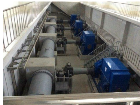
800 kW Booster Pumps
