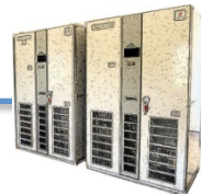
Power conditioners DC -> AC
